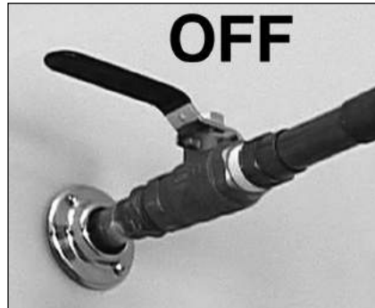
Figure 19 - Cold water supply in off position.
