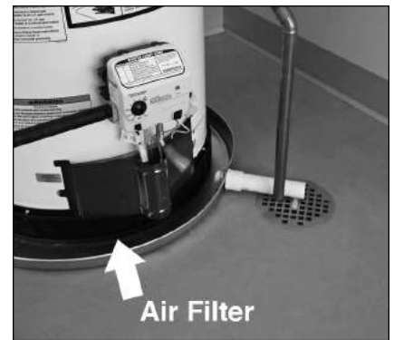
Figure 24 - Filter attached to water heater.
