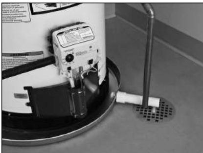
Figure 23 - Metal drain pan piped to drain.
