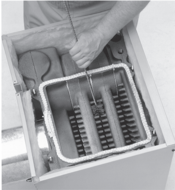
Figure 22 Thoroughly clean flueways between all pins at all angles. Start on top of boiler, finish from the bottom.
