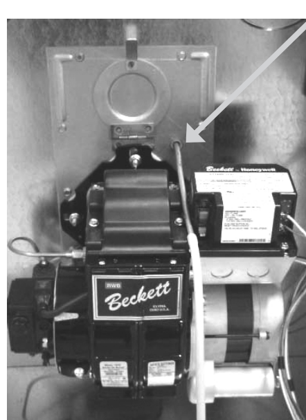
Over-fire draft access port.
