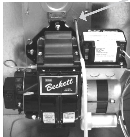
Over-fire draft access port.
