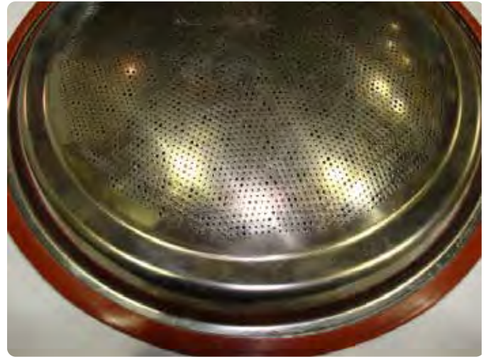
Figure 148 Inspecting exterior and cleaning the burner
