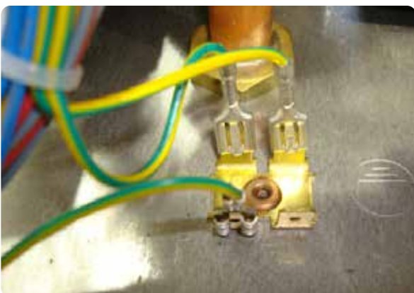
Figure 143 Ignition electrode grounding
