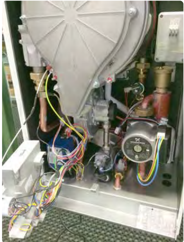
Figure 144 Boiler front panel removed
