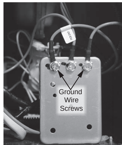
Figure 54 - Location of ground wires
