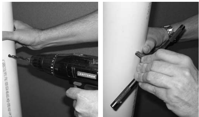
Figure 9.1: Drill and Tap Combustion Test Port
